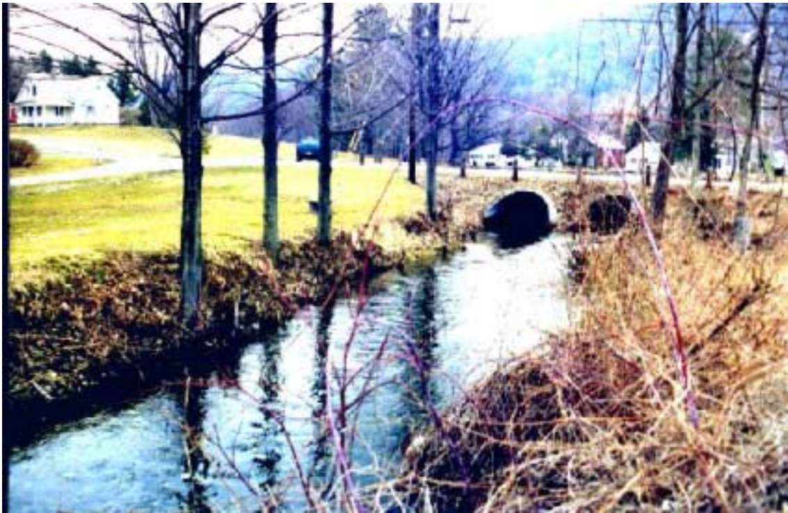
Figure 3. Photographs of the Lake St. Catherine outflow. (a) View of the dam and the start of Mill Brook, taken from across Lake Hill Road. (b) View of the culverts where Mill Brook passes under Lake Hill Road, looking upstream. Both photos taken during high flow, March 19, 1998.
