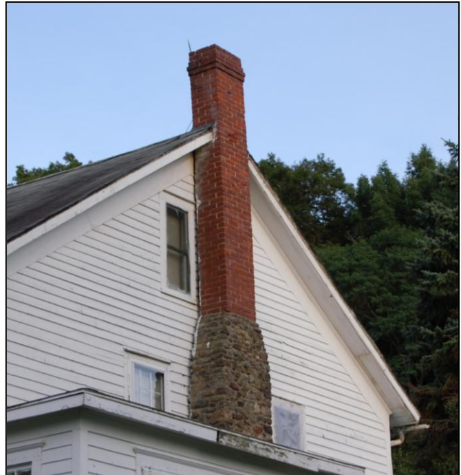
The attic of this house contains a maternity colony, as evidenced by the brown staining next to the chimney at the peak of roof.
